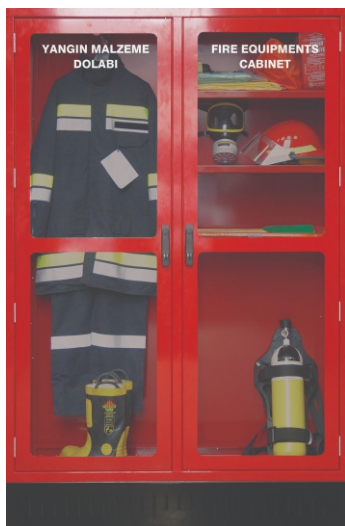
FIRE EQUIPMENT CABINET
