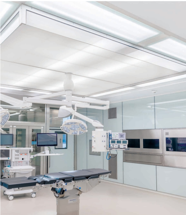
OPERATING ROOM HEPA FILTER
